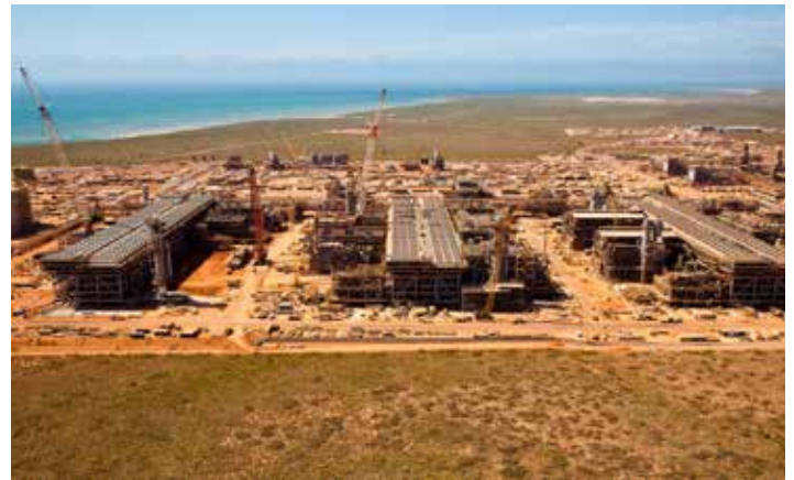
Three LNG production units, known as "trains," at the Gorgon facility
